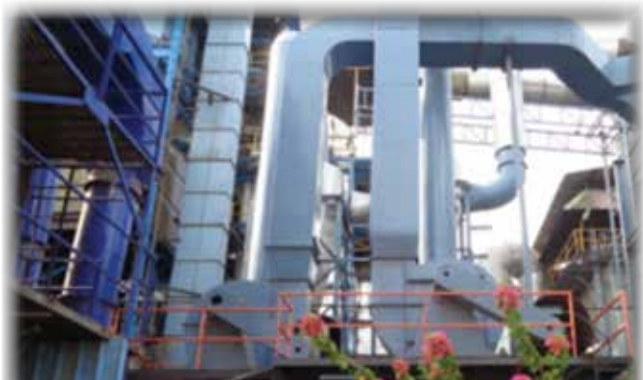
Boiler Area of Co-Gen Plant in MIL-Hapur
